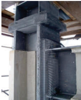
Instalación Contorno XR701
